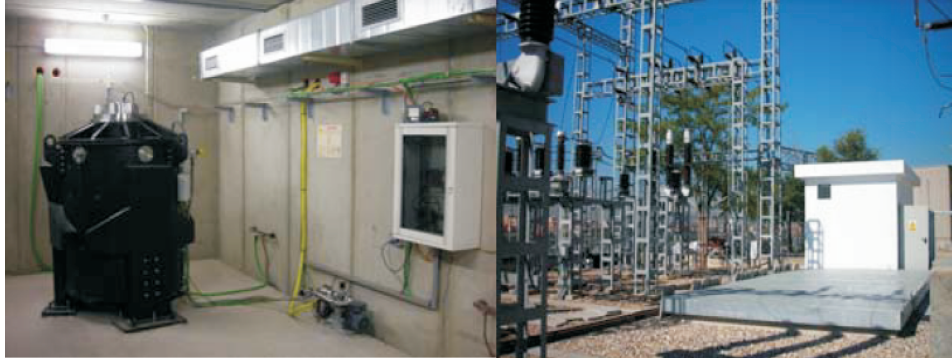
Fig. 28. Substation along the largest railway high-lines
